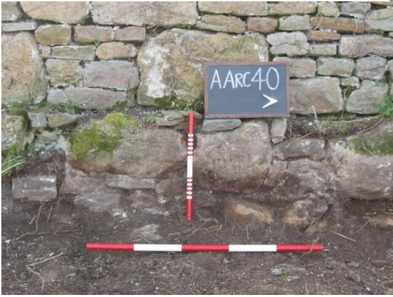
Photo 4 ENE Face of Modern Site Boundary Wall (Scales 1 x 1m & 1 x 500mm)
